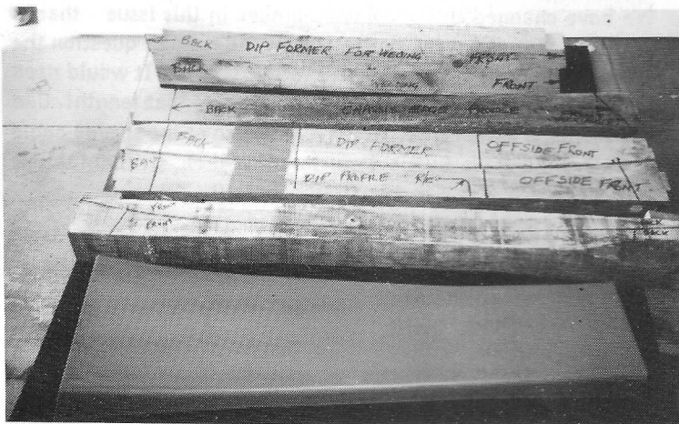
"Timber formers used to make metal work with completed metal in primer in foreground."
