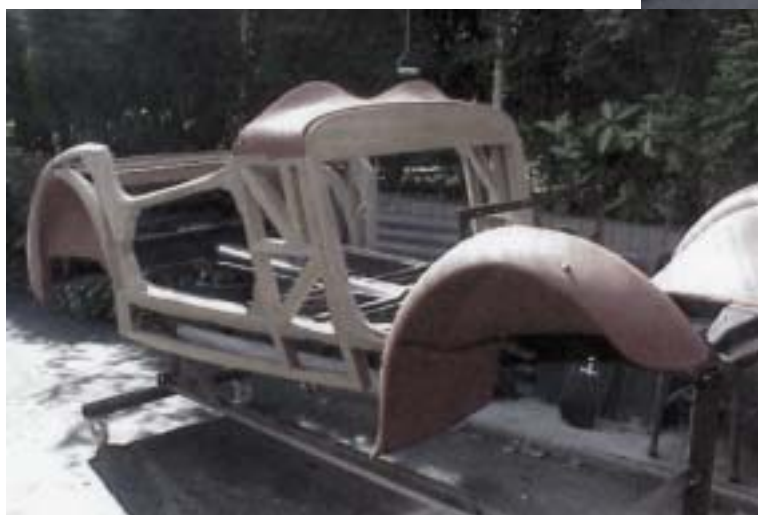
Situation as at June 2003. Note new scuttle with twin wind cowls and completed second front wing.
