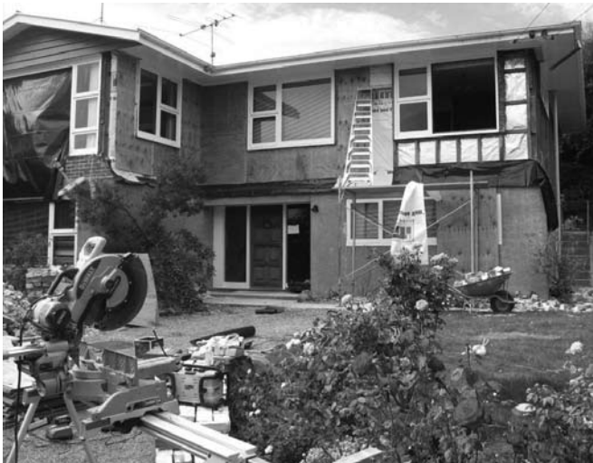
Work is proceeding on making Jill Peter's house habitable, especially through the winter. The bricks not already dislodged by the earthquake have been removed to allow plywood sheets to be placed over the wooden frames of the house.
